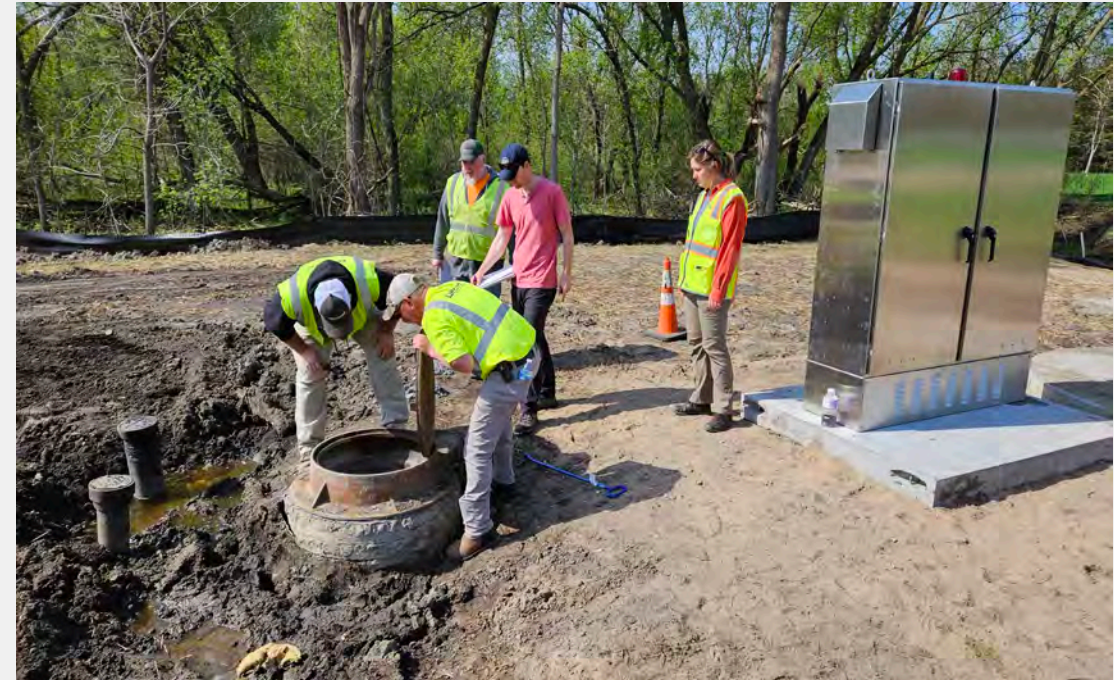
Spring site visit with the Contractor to discuss remaining “punch list” items needed to complete the project.
