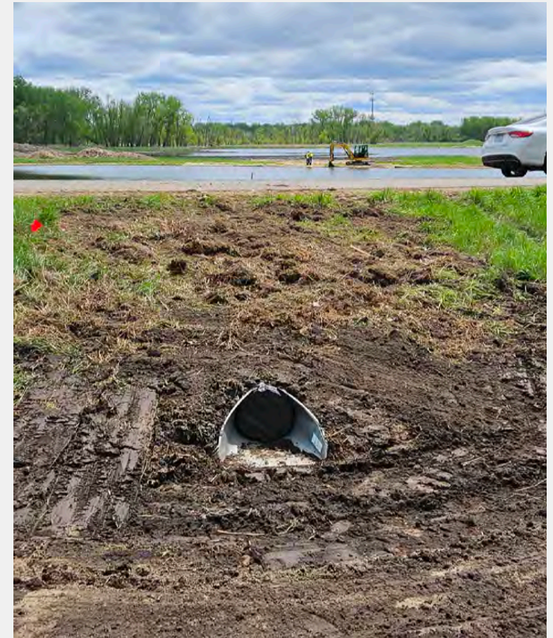
Ditch connection under Hwy 61 and touch up work (background) at the Sunrise River Hwy 61 Wetland Project 5-18-23.
