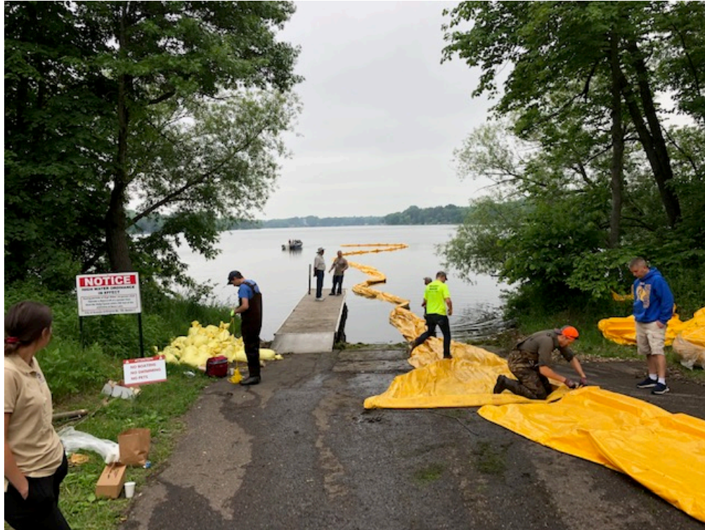
Figure 4 – Zip Tying Sections of Barriers Together as They Are Pulled into the Water
